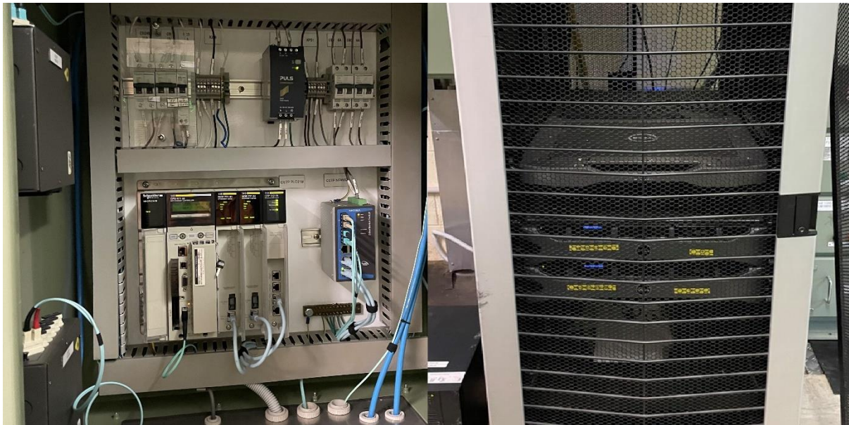
Figure 23. Put hardware (left) and servers (right) in locked cubicles or racks.
