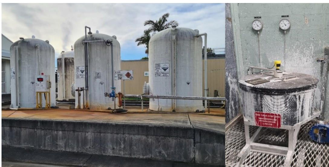
Figure 16. Make pressure washing the preferred option to clean equipment, rather than chemical treatments. MHL tanks (shown right) are messy, so provide splash shields.
