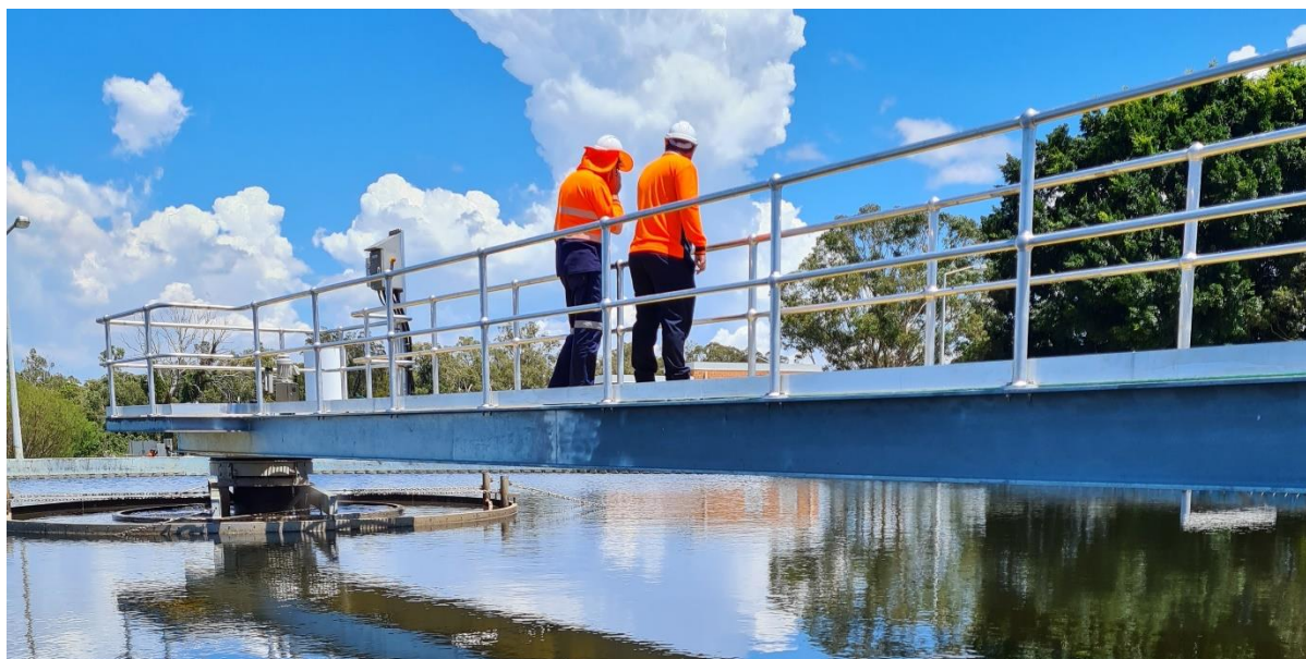
Figure 1. Decisions made during the design of clarifier walkways significantly reduce risks.
